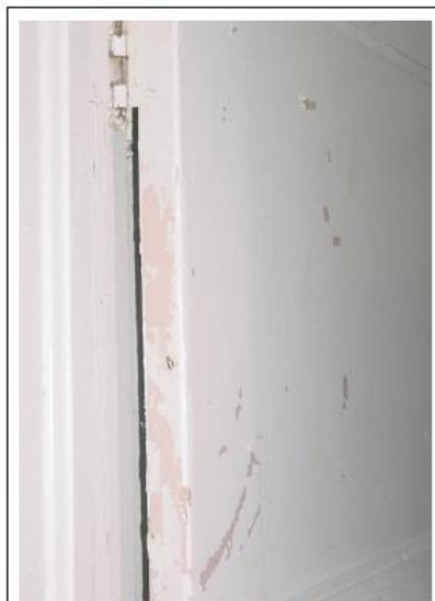
FIGURE 5.7 Impact surface on door and frame.
